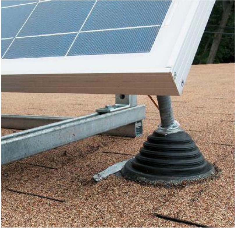
An EPDM rubber boot seals off the opening where the PVC conduit carrying the feed wires penetrates the roof.
