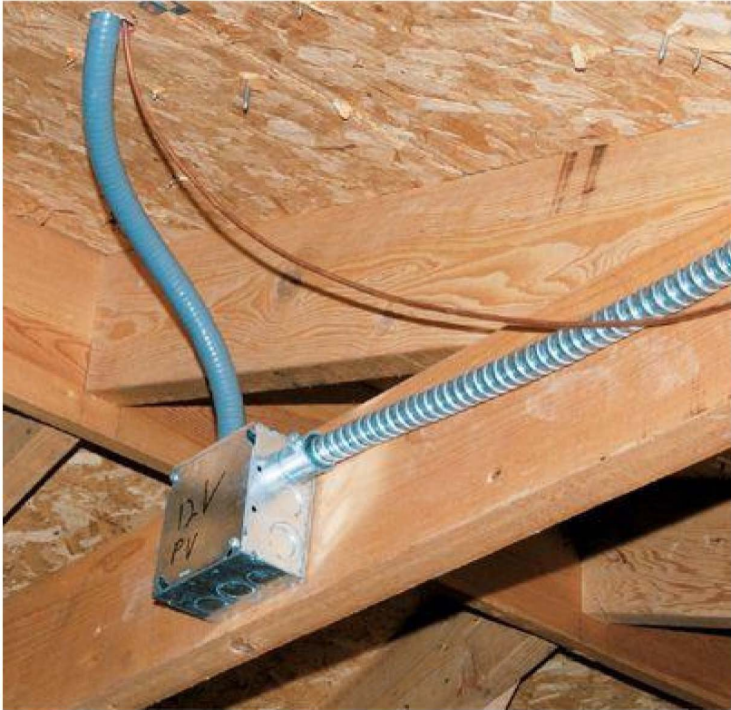
The feed wires from the collector are fed into a junction box inside the structure where connections to the power distribution equipment are made.
