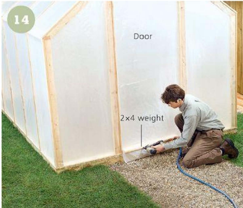
14 Make and hang a door. We simply cut a piece of sheet plastic a little bigger than the opening (32") and hung it with retainer strips from the header. Attach a piece of 2 × 4 to the bottom of the door for weight.
