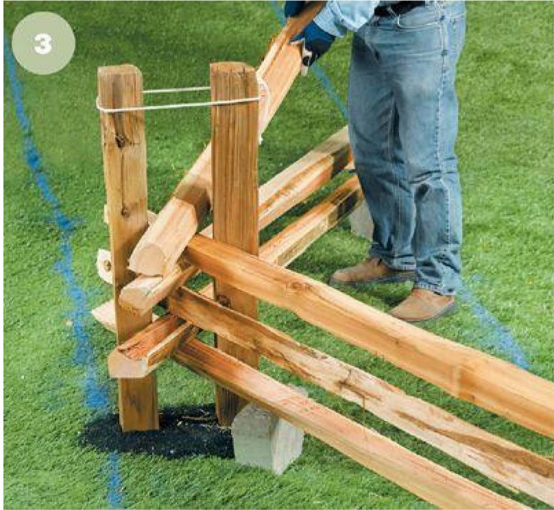
3 Install split fence rails in alternating courses at each post pair, keeping the overhangs even.
